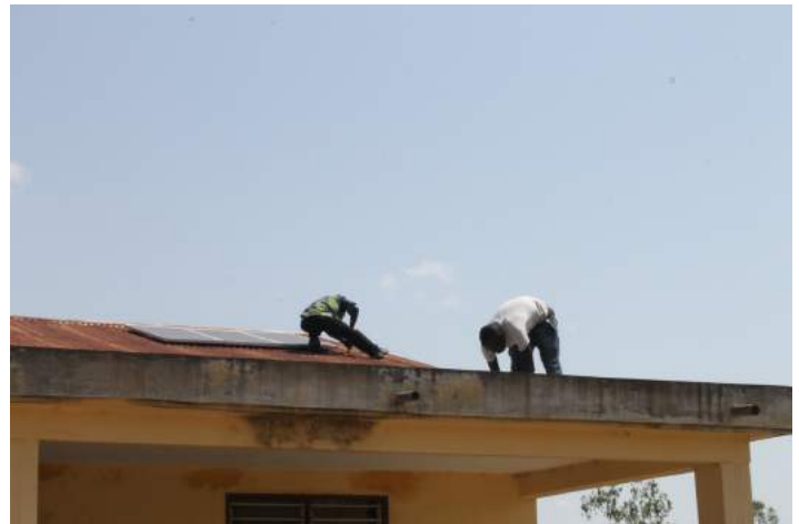
Solar technicians setting up to mount the solar panels on the Kpindi Clinic's roof
