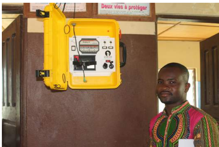
Kpindi Clinic's head nurse, Ayi-Ata Kuevy, next to the newly installed solar suitcase.
